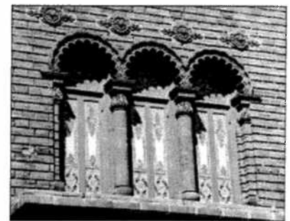
The Medinah's sculptural, monumental quality is enhanced by its decorative terra cotta and distinctive brickwork. Each of its "superbricks" (detail, top) is actually composed of two or four regularly sized bricks. Their "wire-cut" finish complements the building's Islamic-style ornament (above).
